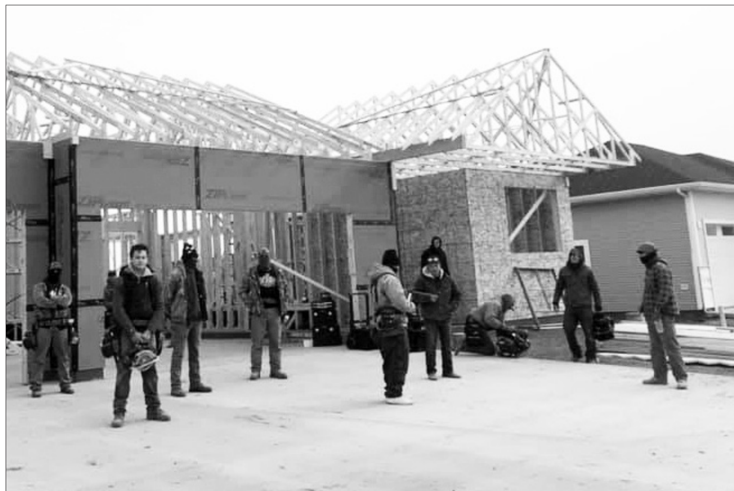
Carpentry students in October 2020 standing in front of the house having installed the walls. The project began in last fall and is now available for sale. (Photos Provided)
